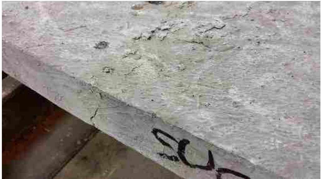
Figure 6.39. Tensile crack on panel SUC3
