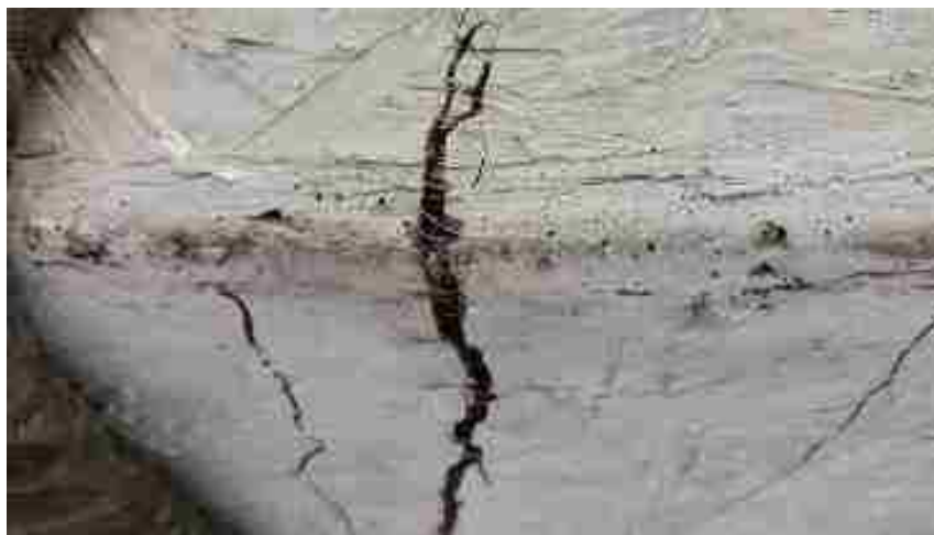
Figure 6.44. Tensile crack on panel SUN3
