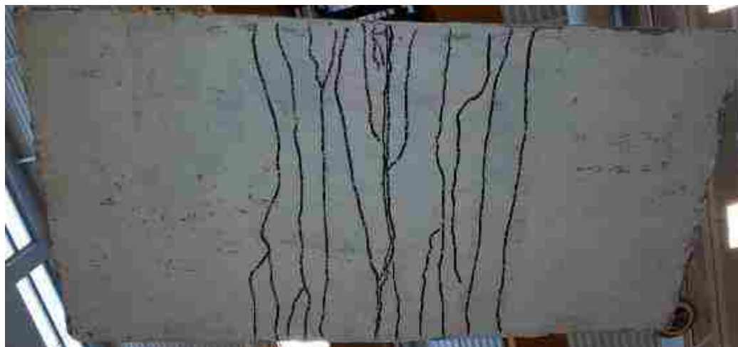
Figure 6.22. Crack pattern formation at the tension face of panel FUW2
