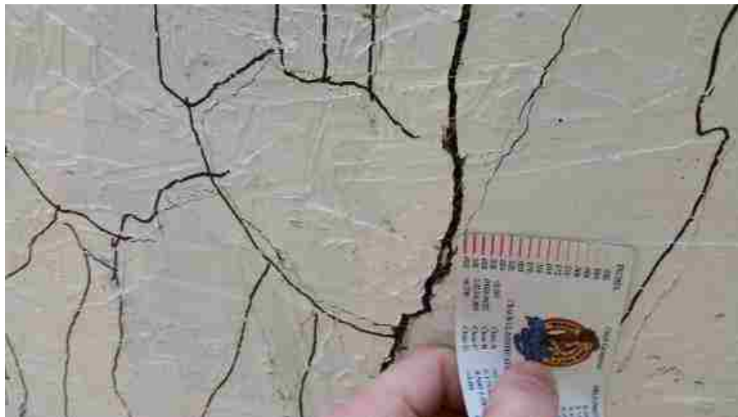
Figure 6.51. Crack widths at the tension face of panel SUC2
