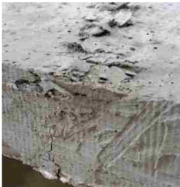
Figure 6.49. Tensile crack on panel SUC2
