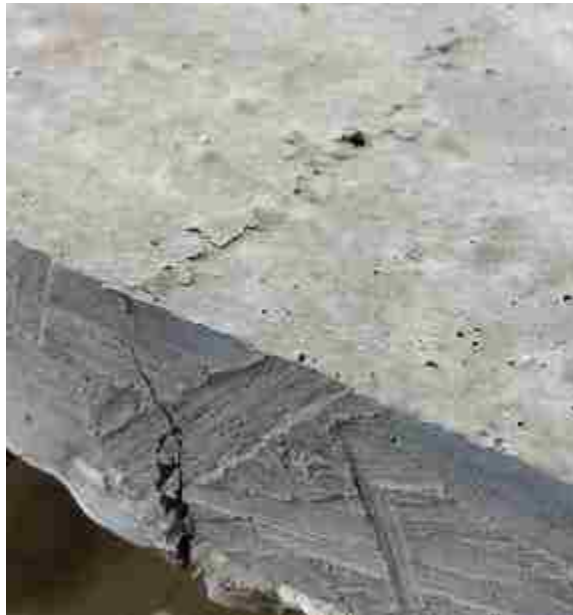
Figure 6.55. Tensile crack on panel SUN2
