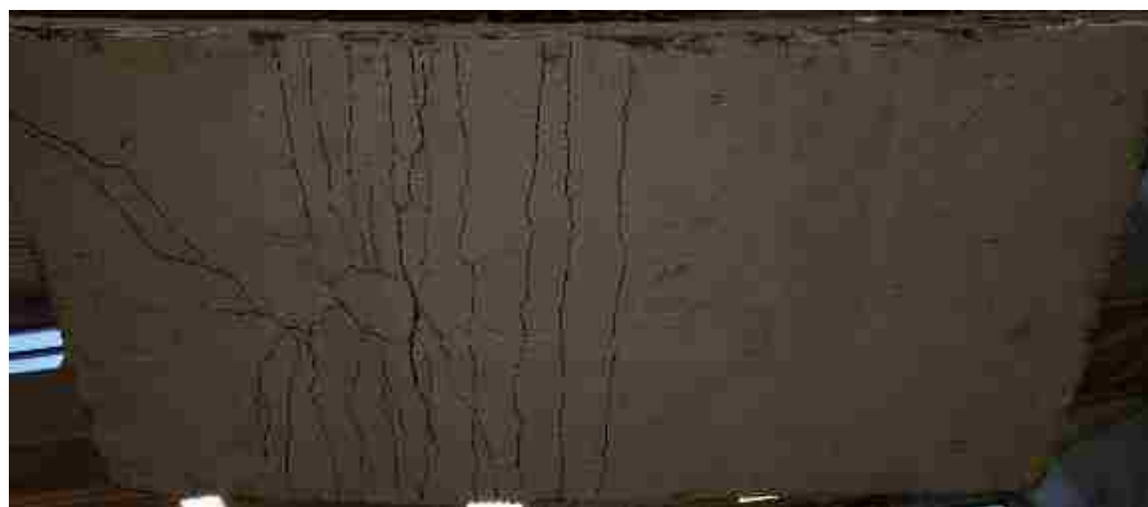
Figure 6.50. Crack pattern formation at the tension face of panel SUC2
