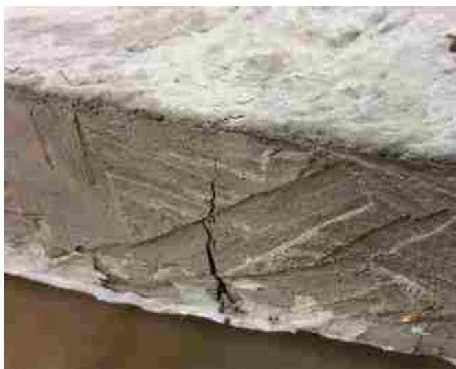
Figure 6.26. Tensile crack on panel FUN2
